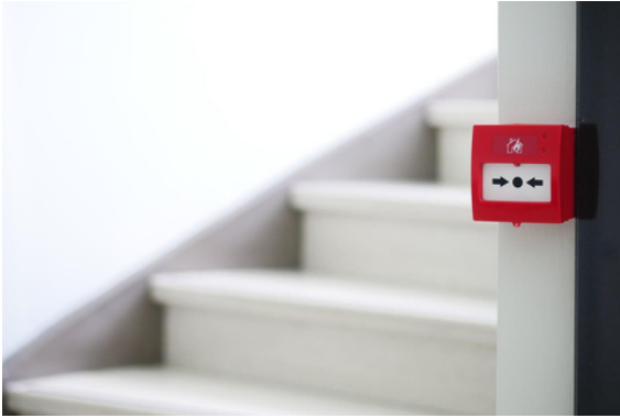
Fire Alarm System
